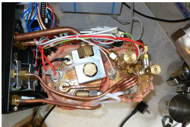
Top of the boilers with hi limit stats, vacuum breakers and safety valves
