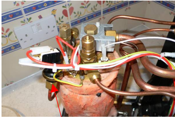
Top of the boilers with hi limit stat, vacuum breaker pressurestat and safety valves
